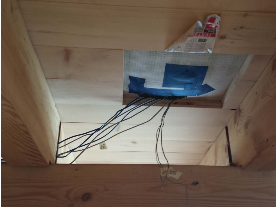
Center Roof Sensor Location
